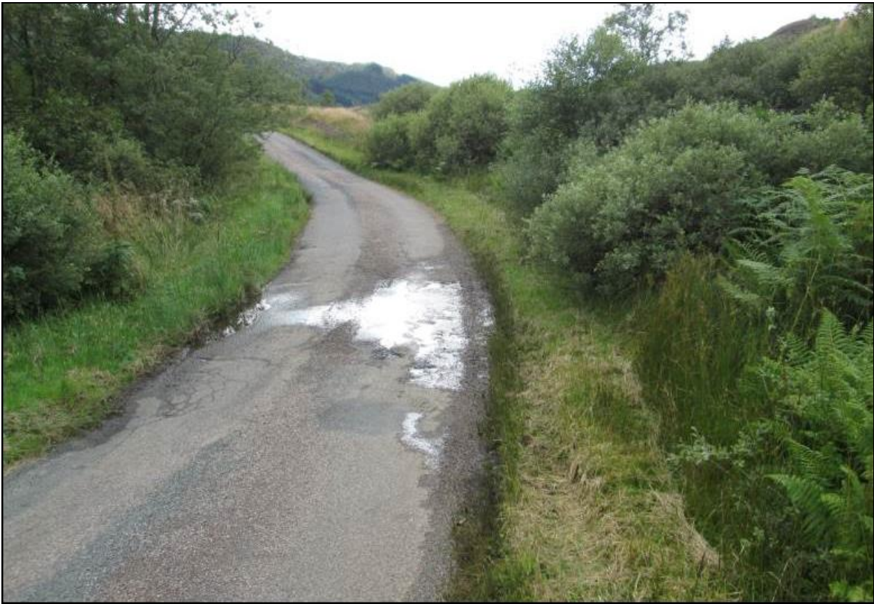
Figure 3.13b Photo Showing Consequences of Inadequate Preventative Maintenance
